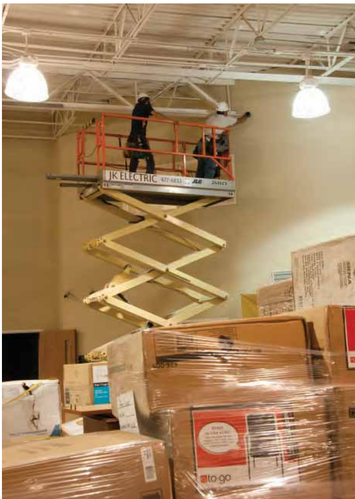
Through the year construction crews and pallets of furnishings heightened CFPIN's anticipation of the new conference center.
